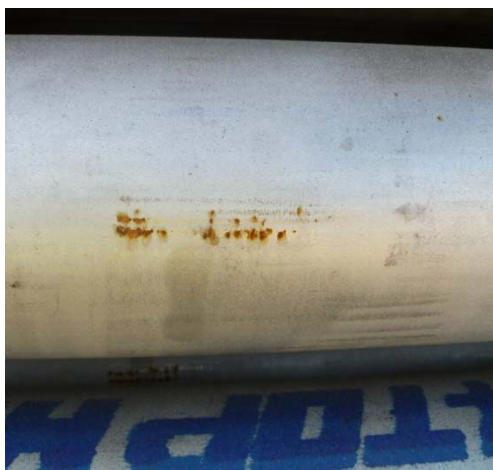
Pic # 1 Superficial contamination
